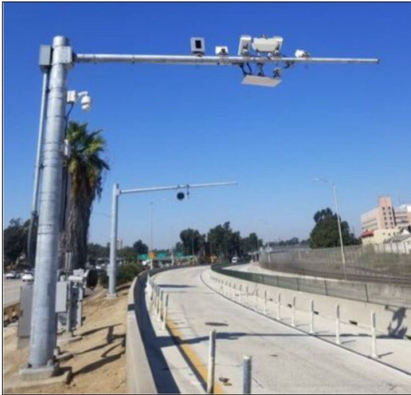
Figure 7-7. Occupancy Detection System installed on I-10
