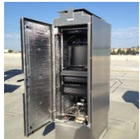
Figure 7-2. Typical Lane Controller Cabinet
