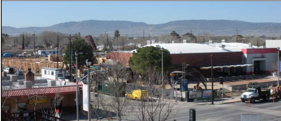
Sagebrush Apartments and Bex Bar and Grill, featuring prominent plaza areas, under construction.
