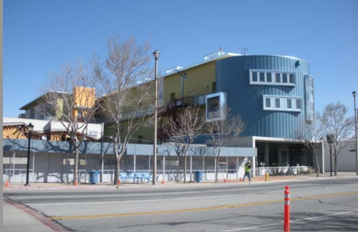
Lancaster Museum and Art Gallery under construction adjacent to existing artist lofts.
